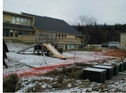
This innovative/alternative system behind the Town of Warren's elementary school is one of several EPA demonstration grant projects that Stone has completed.
