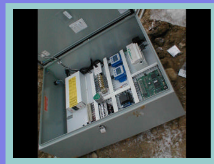
Remote Monitoring Control Panel
