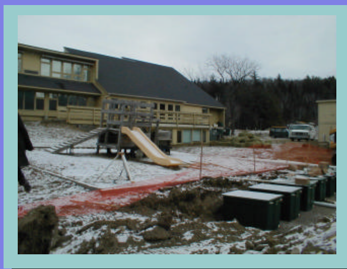
Treatment System Behind School
