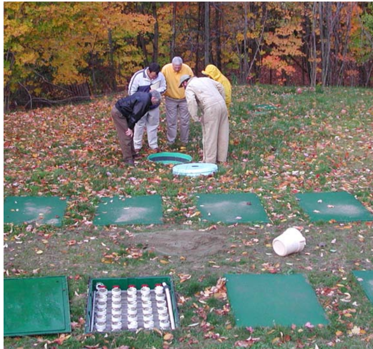
Septic systems that use alternative technology, such as this textile filter system, generally require regular maintenance that can be included in a management program.
