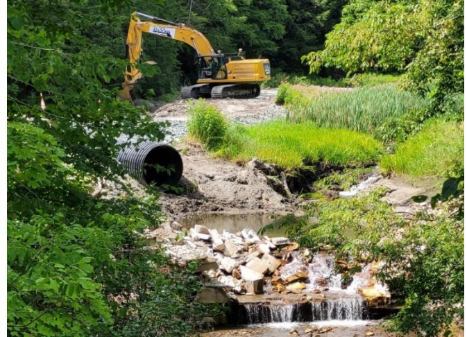
Breached face of the Pelletier Dam and impoundment (August, 2022)
