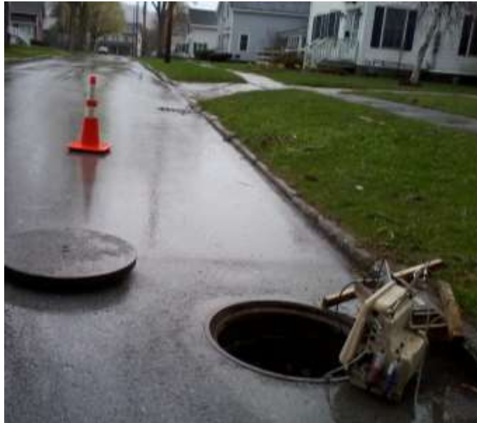
Manhole on Rugg Street in which flow monitoring equipment was deployed, St. Albans, VT.
