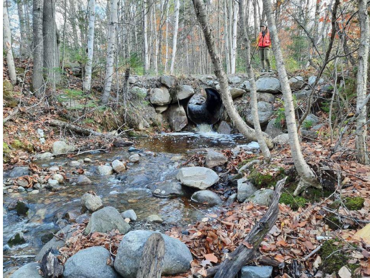
Downstream channel showing aquatic organism passage barrier at Alder Brook in Success, NH
