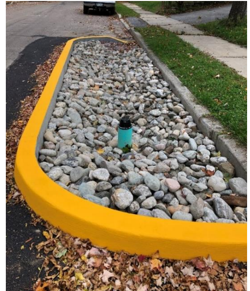
Curb extension bioretention feature on Pine Grove Terrace, after construction and prior to planting.
