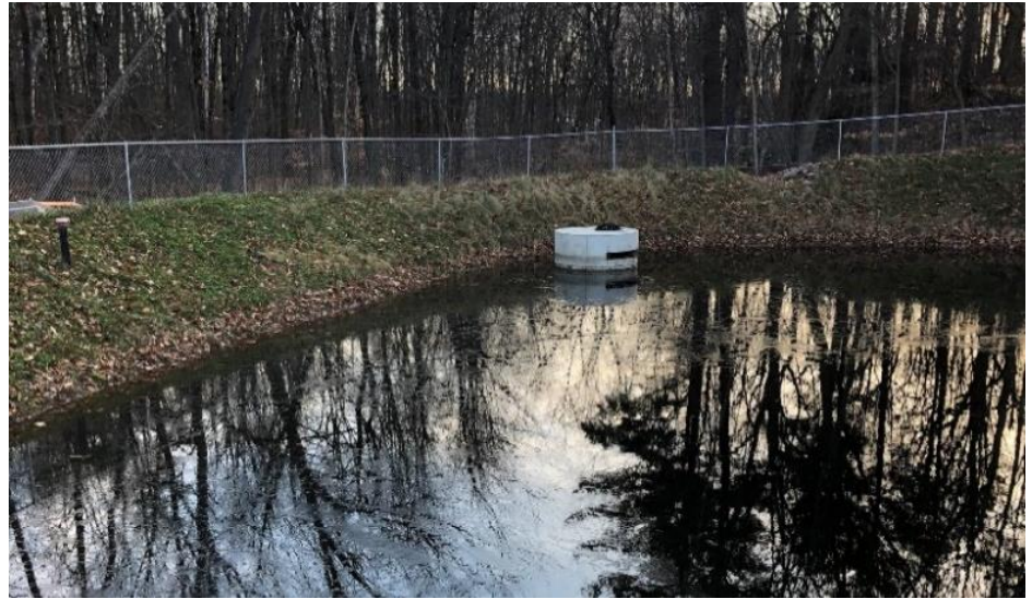
Final conditions of the pond at the lower portion of the Pine Grove Terrace drainage area and cul-de-sac.
